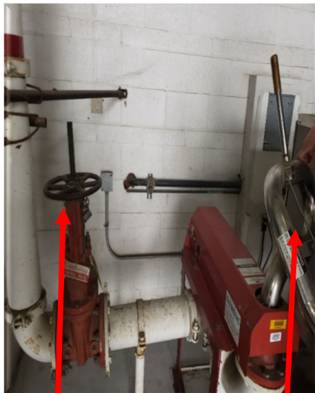
Manual Shut Off Control Valve (turn clockwise)
